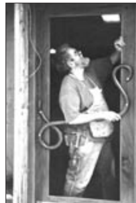
Jeffrey Briggs installs his masterpiece – the new front door to the Sargent Gallery.
