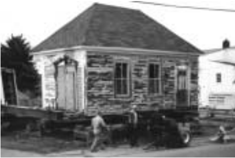
The NAA annex to be moved, placed on its new foundation, and renovated
